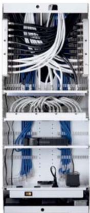
Structured Cabling Cabinet
